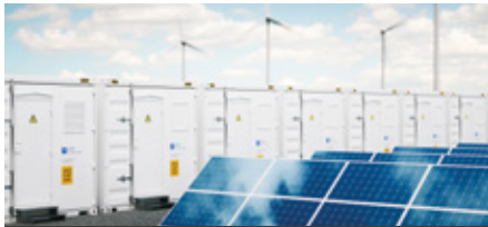
Battery energy storage systems (BESS)
